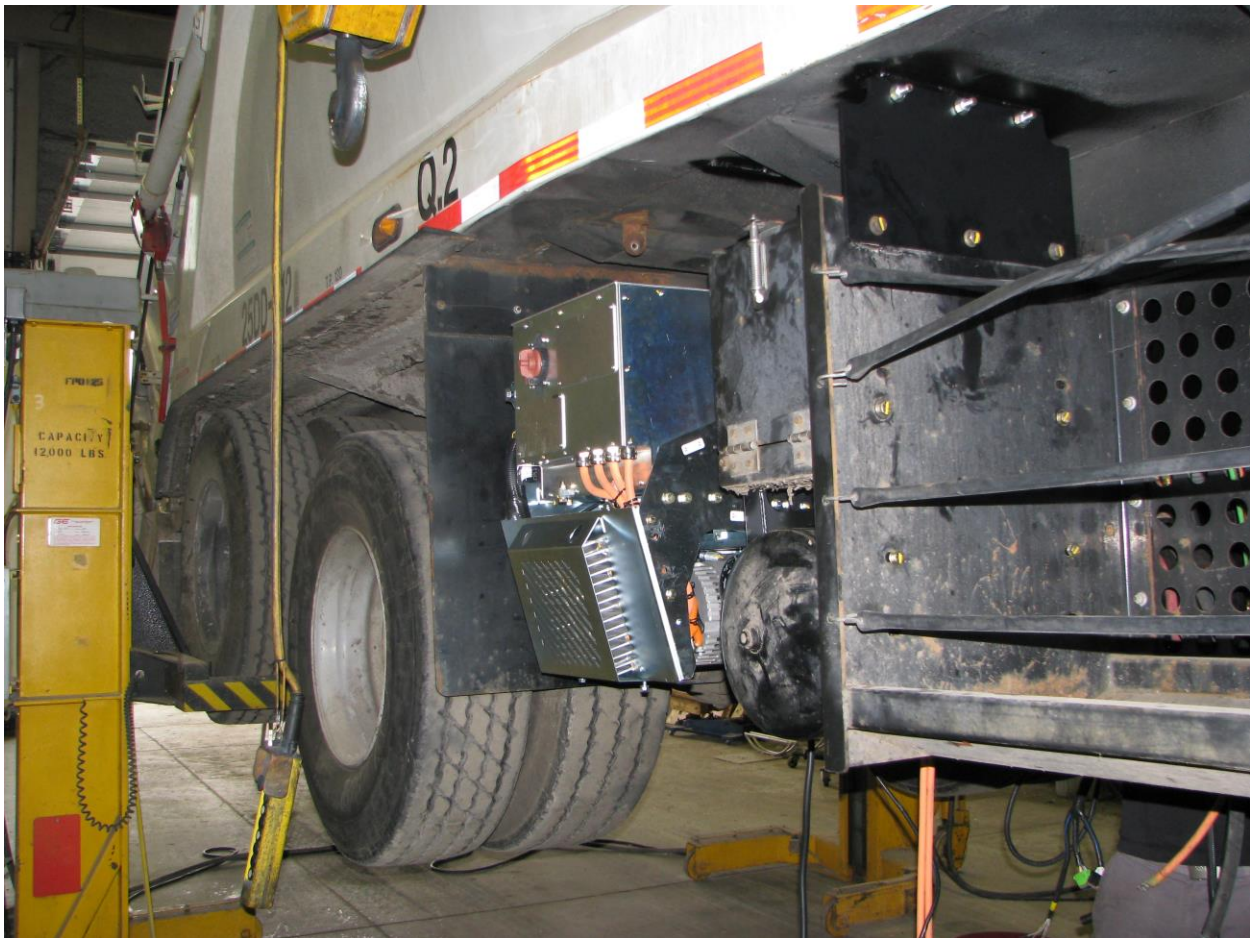
Power pack installed on the vehicle without covers / enclosure
